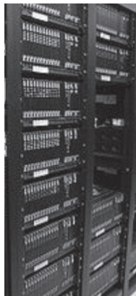
Figure 6.7: Modem Bank at an ISP
